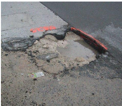
Pothold located on Braddock Avenue near Reinwald's
