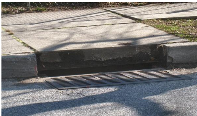
Cast iron curb section of this catch basin has been stolen.
