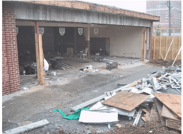
Cedar Lane interior is being gutted. It is anticipated that the building will probably be totally torn down.
